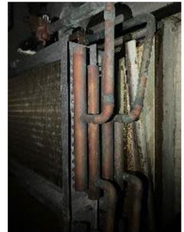
Image 2: Failed Heat-Recovery Coil
