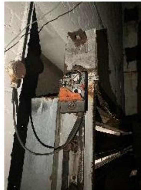
Image 1: Derelict variable intake Louvres
